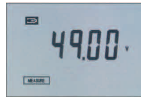
Voltage Measure Display
