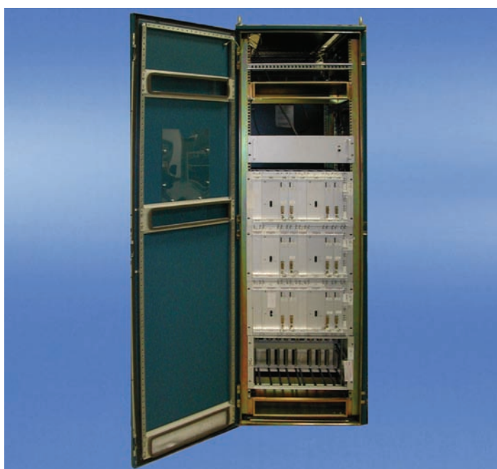
Application: Control system
