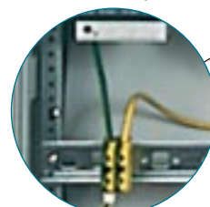
Surge arrester / Earth terminal
