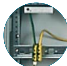
Surge arrester / Earth terminal
